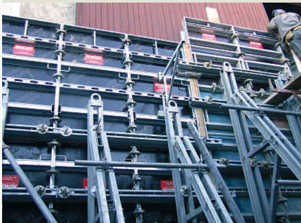
ST 2000 Project "BIOENERGIE STRASSER" Neukirchen, Austria
